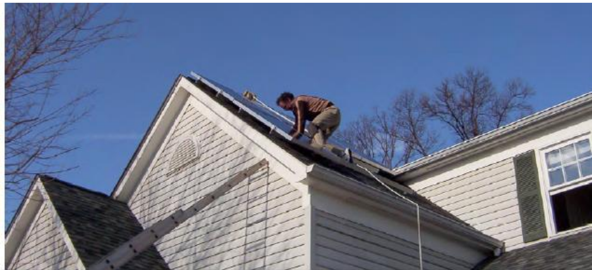
Figure-9: Mounting the fifth panel. The hoisting jig can be seen at the top of the roof and the rope used to pull the panels up onto the rails is currently not in use behind me.
